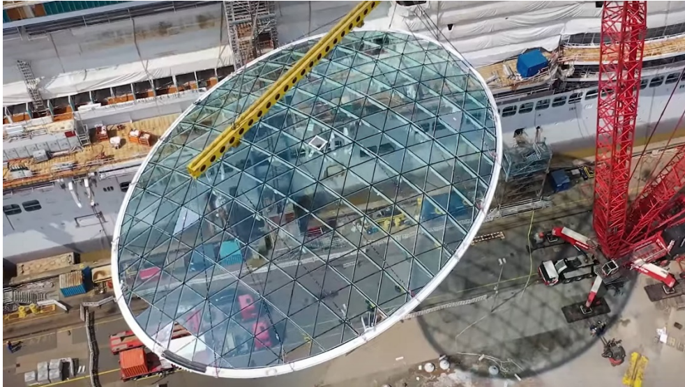
Fig. 2 P&O glass dome Iona is the first structure of this type in the cruise ship industry. Designer: Martin Francis | Structural Engineers: Eckerlesley O'Callaghan | Shipyard: Meyer Weft
